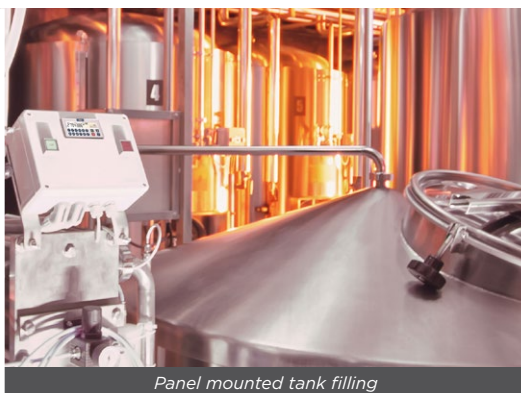
Panel mounted tank filling
