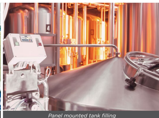
Panel mounted tank filling
